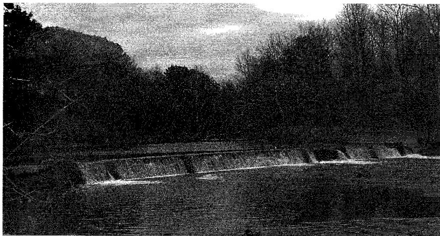
Dam built by Clark Hurd and Joseph Briggs on the Buffalo Creek behind the church.
